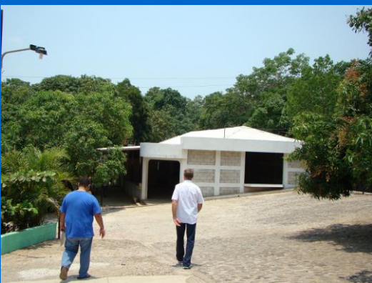
New kitchen at the orphanage that has been under construction for over two years, with work progressing as the funds are given.
